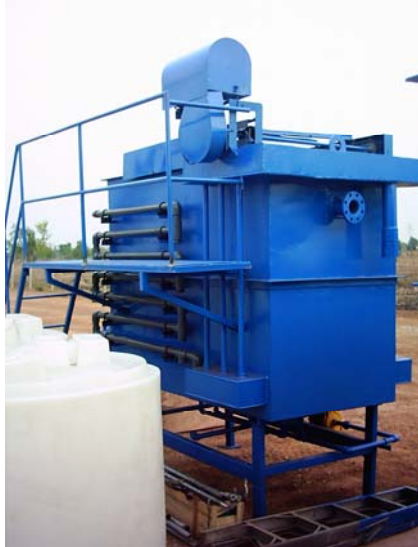
@ Pan Orient Vichienburi Oil Drilling Field CAP. 5 cubic meter /hour
